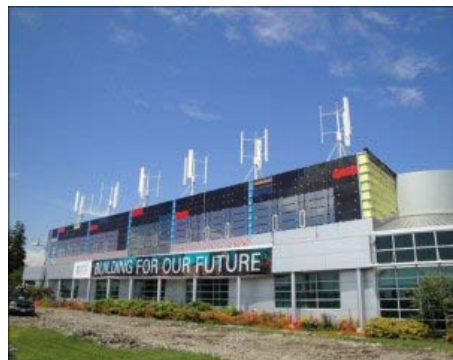
Durham College Installation - Durham College installation of 6 VAWTs, Oshawa, Ontario, Canada
