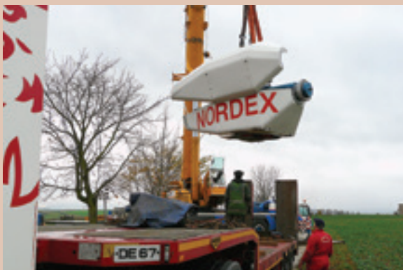
Lowering the nacelle. The turbine and tower were shipped to Northern Ireland where it found a new home. Note image on the tower at left. Many wind turbines in Germany are "adopted" by local groups who paint fanciful patterns on the towers.
